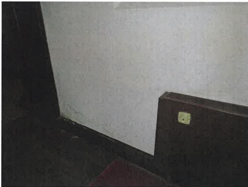
Photograph 20: White substance and stains on the north wall of the church.
