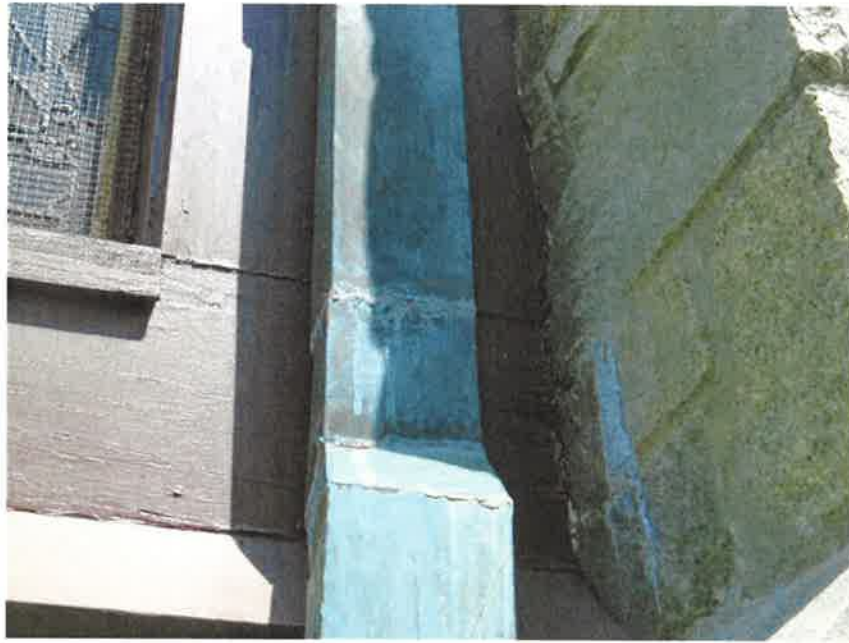
Photograph 17: The wood trim on the west elevation of the altar is rotted and a gap is between the wood and the stone.
