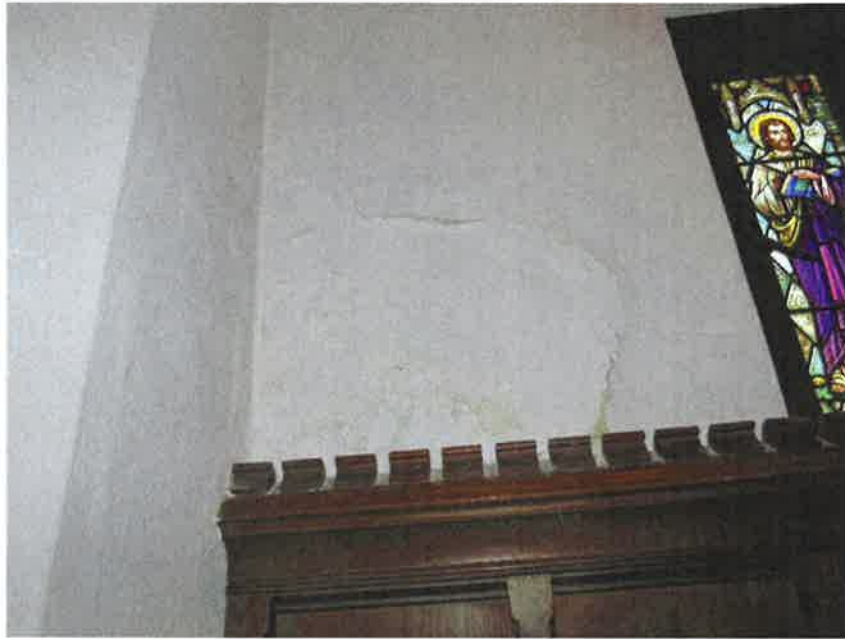
Photograph 21: White substance and stains on the west wall of the altar.
