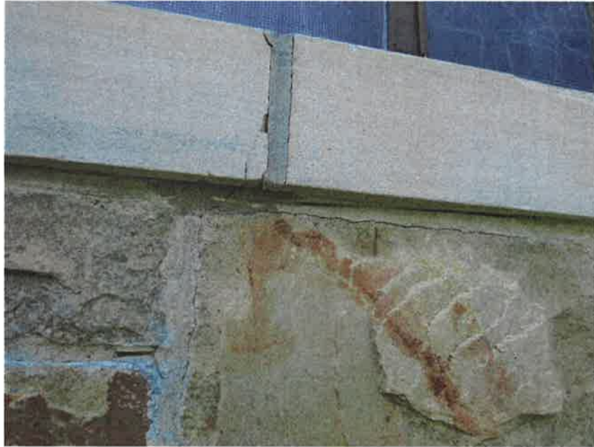
Photograph 3: The mortar is cracked throughout the church elevations.
