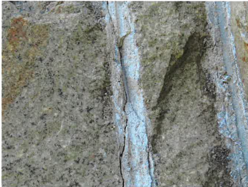
Photograph 4: The mortar is cracked throughout the church elevations.
