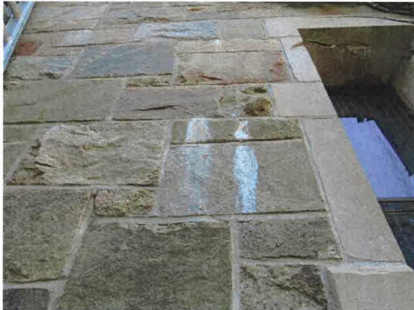
Photograph 14: White stains are on the stones on the east elevation below the bell tower.
