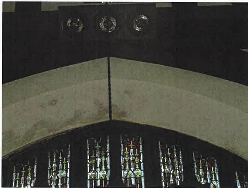
Photograph 18: White substance and stains on the east wall of the church around the stained glass window.
