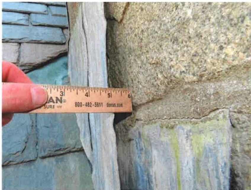
Photograph 12: The roof step-flashing on the sides of the altar are loose and a gap is between the flashing and the north elevation of the church.
