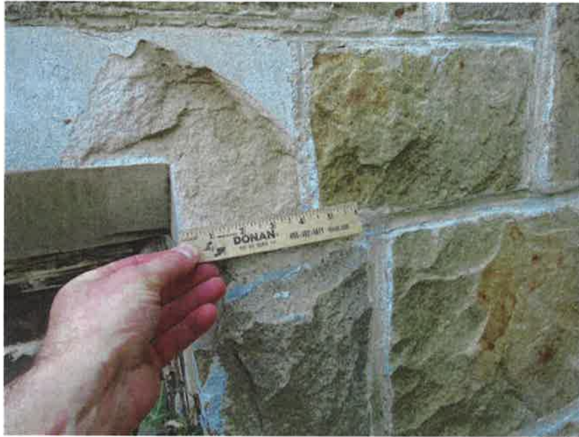
Photograph 7: The stone surrounding the crawlspace window on the east elevation is deteriorated and missing.
