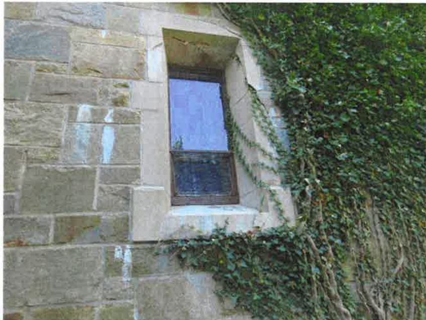
Photograph 16: The stones around the bell tower's east elevation window are cracked, displaced, and deteriorated.
