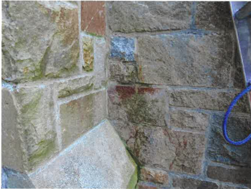
Photograph 15: Water is leaching out of the stone on the east elevation of the bell tower.
