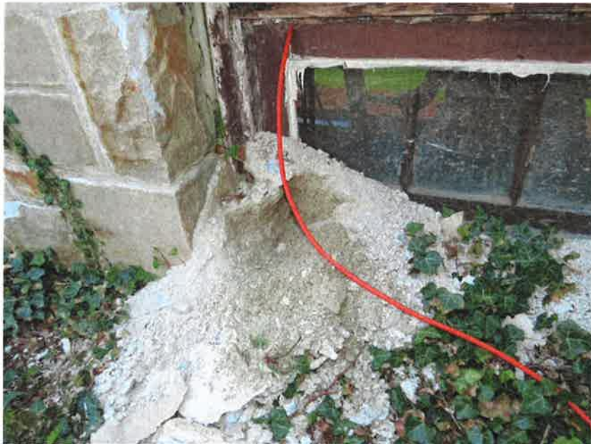
Photograph 6: Piles of deteriorated and washed-out mortar and stone are below the bottom windows on the east elevation.
