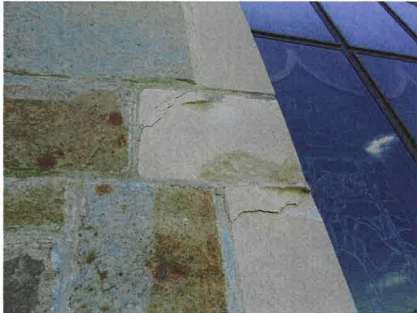
Photograph 11: The stone surrounding the stained glass window on the east elevation is cracked and deteriorated.
