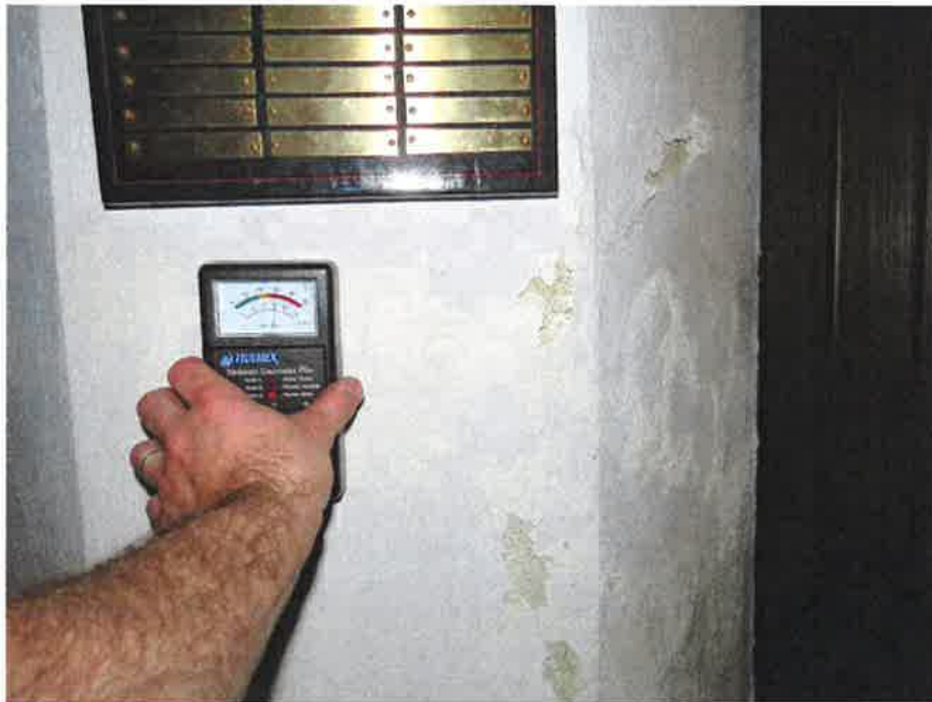
Photograph 22: White substance and stains on the altar's east wall, the reported bell tower's floor drain is within this wall.
