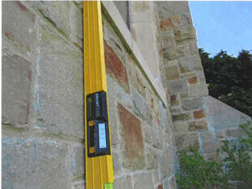
Photograph 10: The stone approximately 3 feet below the stained glass window on the east elevation is bowing outward.
