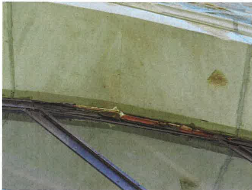
Photograph 8: The wood trim along the top of the stained glass window on the east elevation is cracked and deteriorated.
