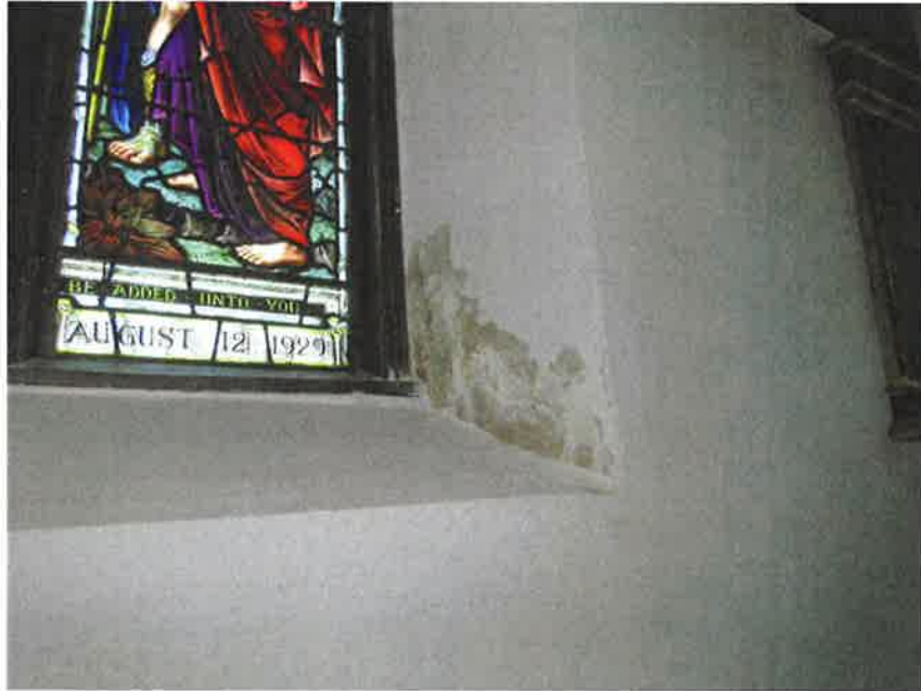
Photograph 19: White substance and stains on the east wall of the church around the stained glass window.
