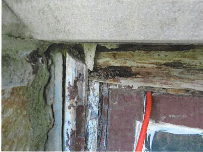
Photograph 9: A gap and deteriorated wood is around the crawlspace windows on the east elevation.
